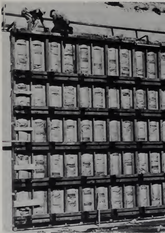
Figure 174.—Form insulation for protection of concrete. This is a reliable method that avoids heating PX-D-33054.
